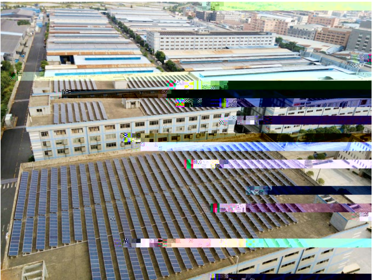
Solar PV Panels on the Roofs of Lesso Plants
