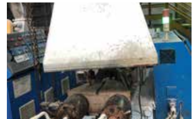
Exhaust gas treatment device in a workshop
